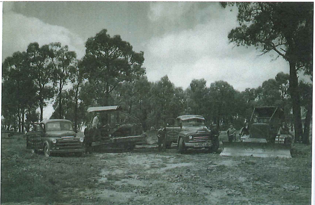
Pictured: First day of work on the new Lords Raceway track by A.L. & B.G. Pearce
